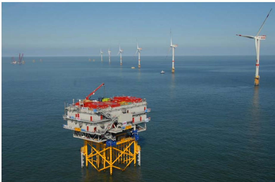
Figure 4. The OTS was installed on March 17 th 2012. On the background the six phase I turbines (photo C-Power).
