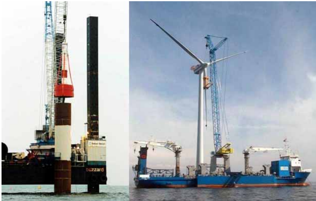
Figure 5 Left: Pile driving from the jack-up rig "Buzzard". Right: mounting of wings from the jack-up "Ocean Ady". Photos : Vattenfall A/S.
