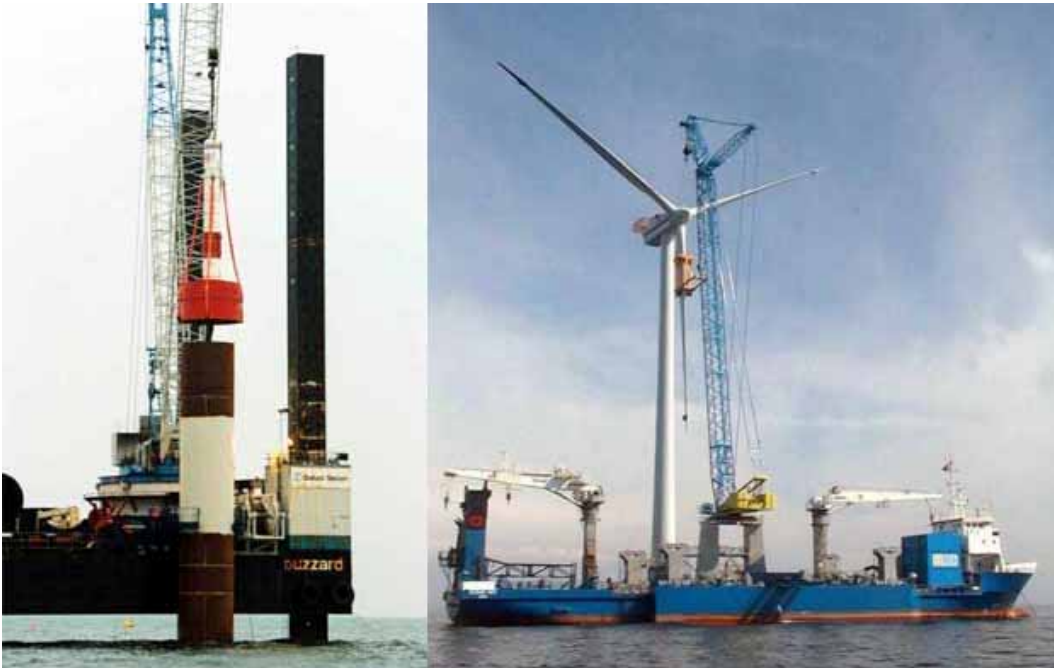
Figure 6 Left: Pile driving from the jack-up rig "Buzzard". Right: mounting of wings from the jack-up "Ocean Addy". Photos : Vattenfall A/S.
