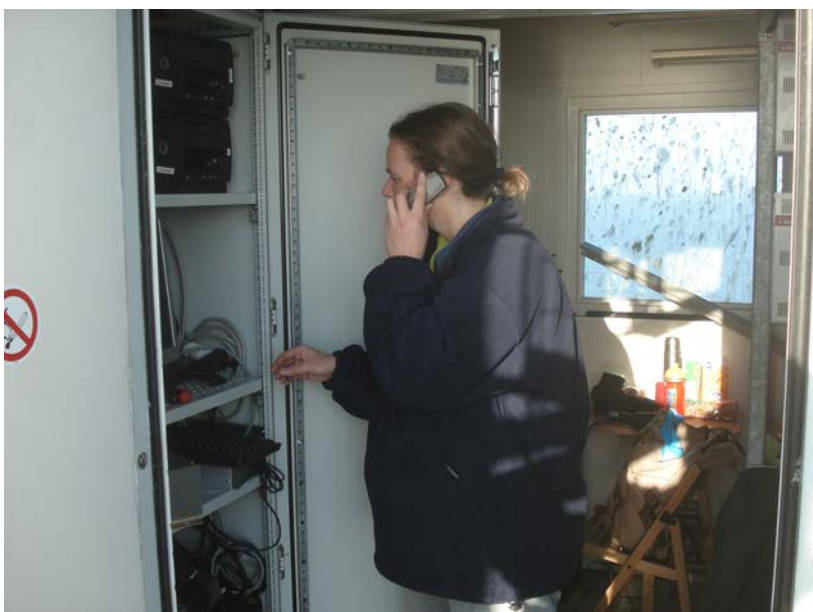
Computer cabinet on the metmast. Note the remains on the window of cormorants resting on the metmast (photo M. Poot).
