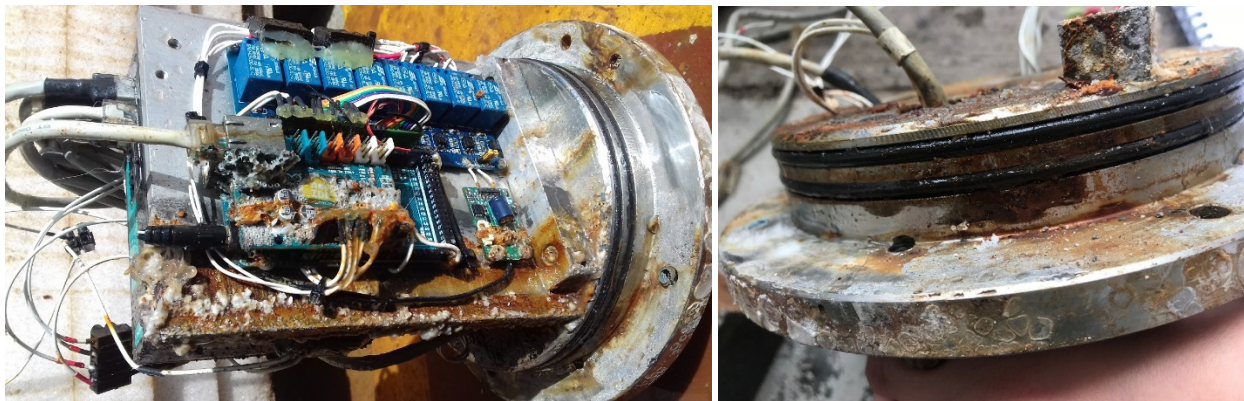
Figure 5. (Left) Electronics inside of the HiCUP junction box were severely corroded. A clear ‘tide line’ is visible allowing the approximate volume of water inside the junction box to be calculated. (Right) Corrosion between the two O-ring seals on the end cap of the junction box.
