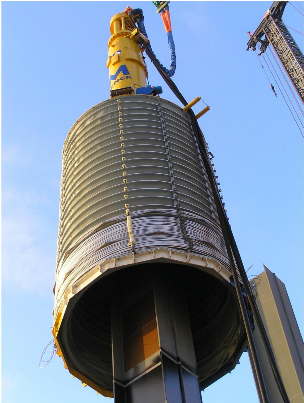
Fig. 4-10: MENCK bellows as surface noise protection system
