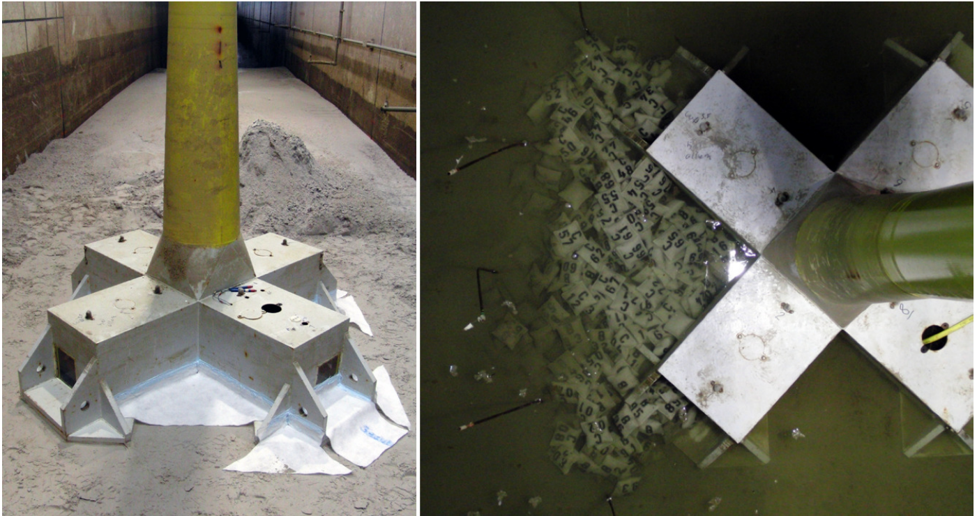
Figure 4-10: Foundation with installed fleece for Variant 2 (left) and foundation during installation phase of the scour protection system (right).
