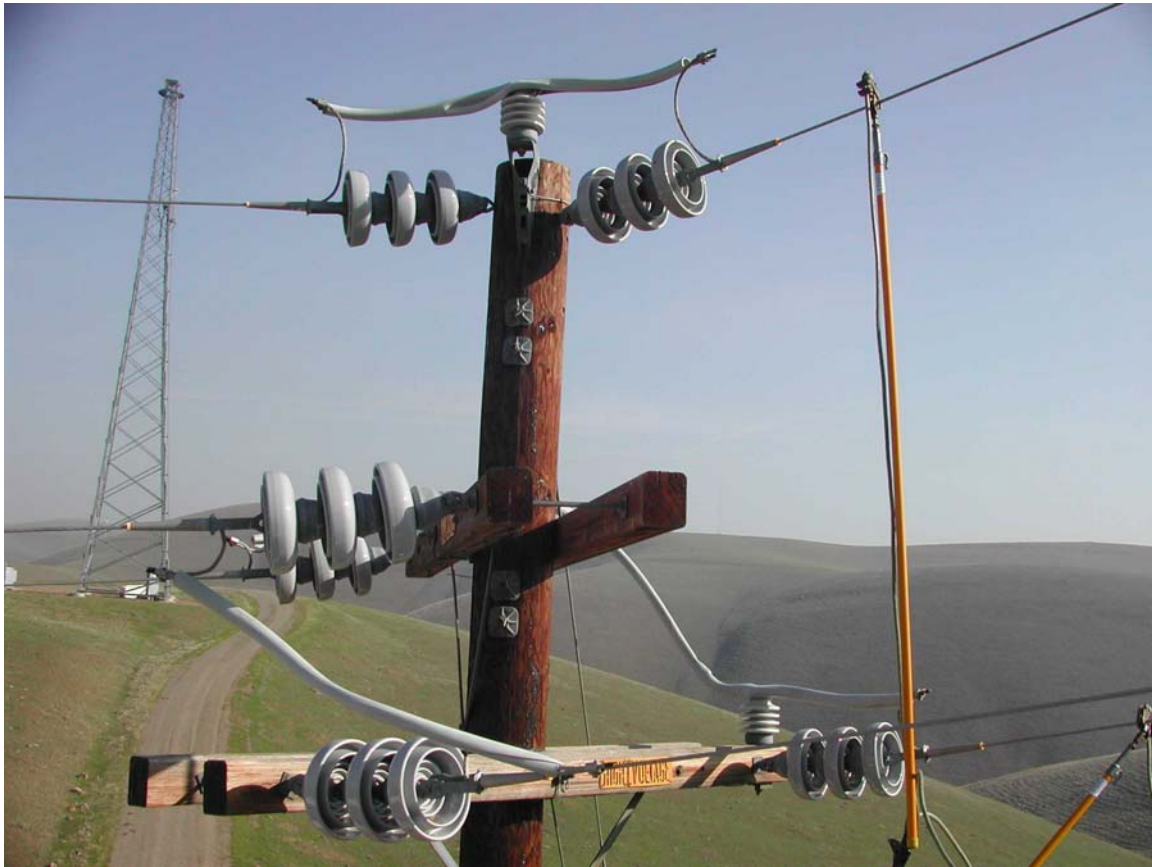
Figure 4. Typical corner pole with insulated wires.
