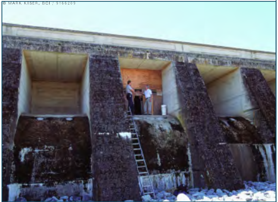
Bob Wisecarver (right) and a helper at the Pardee Dam during the original construction of the “bat cave” about 12 years ago.
