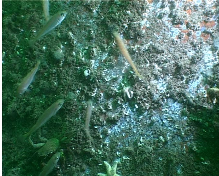
Figure 13 Scour zone on Turbine 30. Note the bare un-colonised patches and the white squiggles of the tube worm Pomatoceros sp. Photograph: F. Bunker
