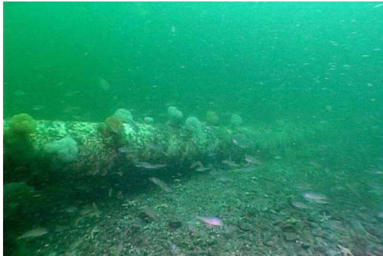
Figure 14 J-tube lying exposed in what may be a scour pit around Turbine 17. Photographer: F. Bunker
