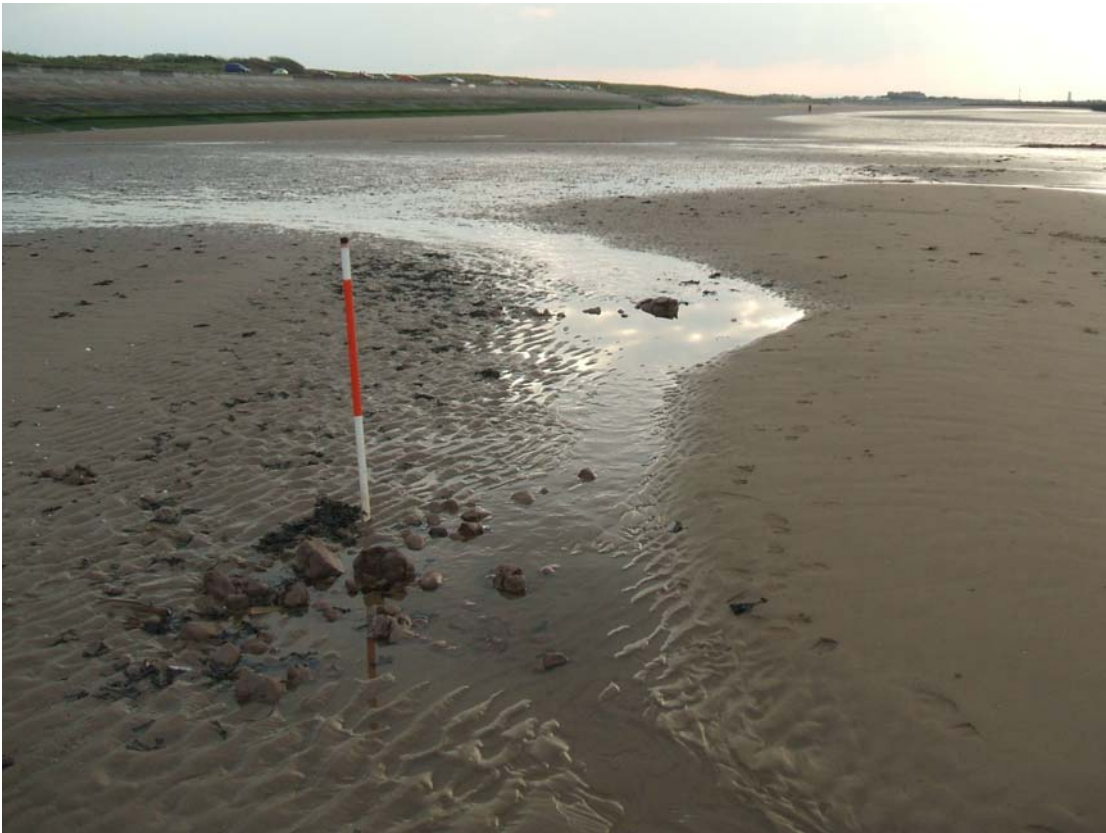
Figure 8. Site 22HDD 19 days after cable exposure and re-burial.
