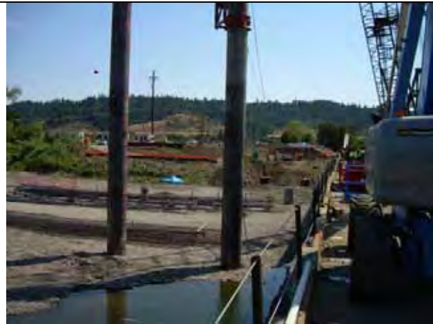
Figure I.3-17b CISS Piles Driven to Support New Geyserville Bridge across the Russian River
