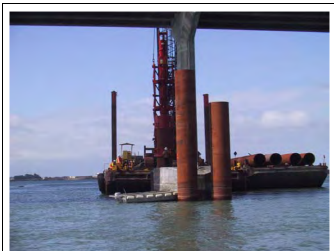
Figure I.11-5 Driving 60-Inch Diameter Piles – Pier S12, Samoa Channel at Humboldt Bay, Eureka, CA
