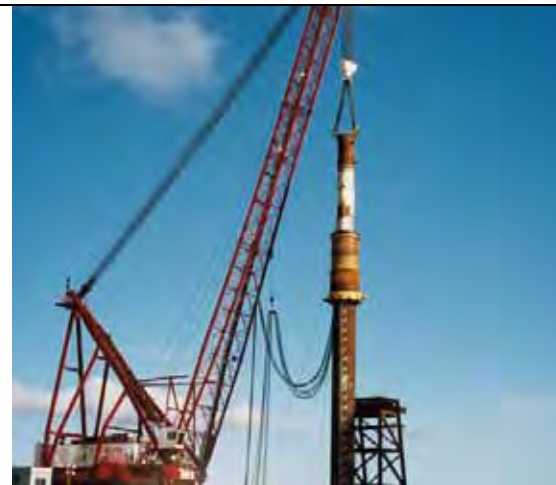
Figure I.9-3b Large Hydraulic Hammer (MHU1700T) Hammer Used for Last Quarter of Pile Driving Where Resistance Was Greatest
