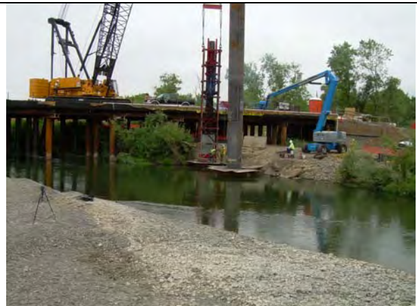
Figure I.3-22b Driving the Top Pile Section of Bent 5 Using a Dewatered Casing to Reduce Sound
