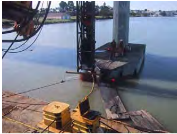
Figure I.11-2a Driving 36-Inch-Diameter Pile in a 5-Foot Casing with Inside Bubble Ring – Humboldt Bay Bridges, Eureka, CA
