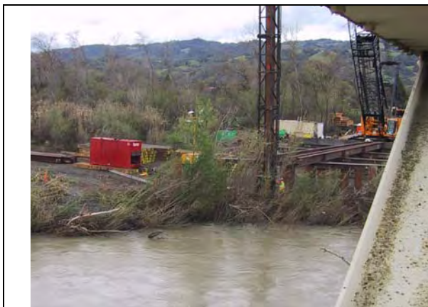
Figure I.3-18a Trestle Pile Driven on East Bank. Note trestle piles extend back several hundred feet.
