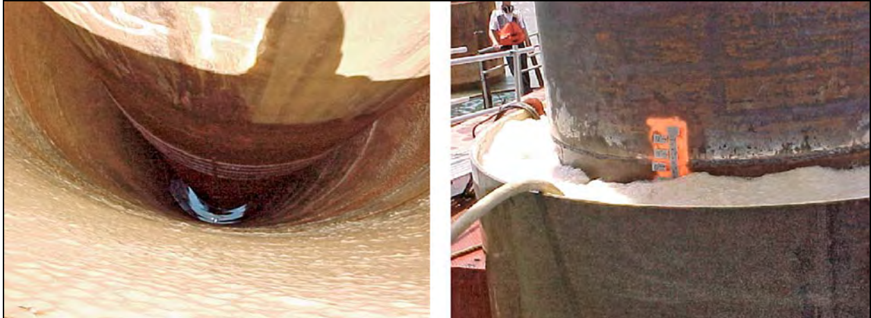
Figure 2-29. Confined Air Bubble Curtain System Used in an Isolation Pile at the Benicia-Martinez Bridge
