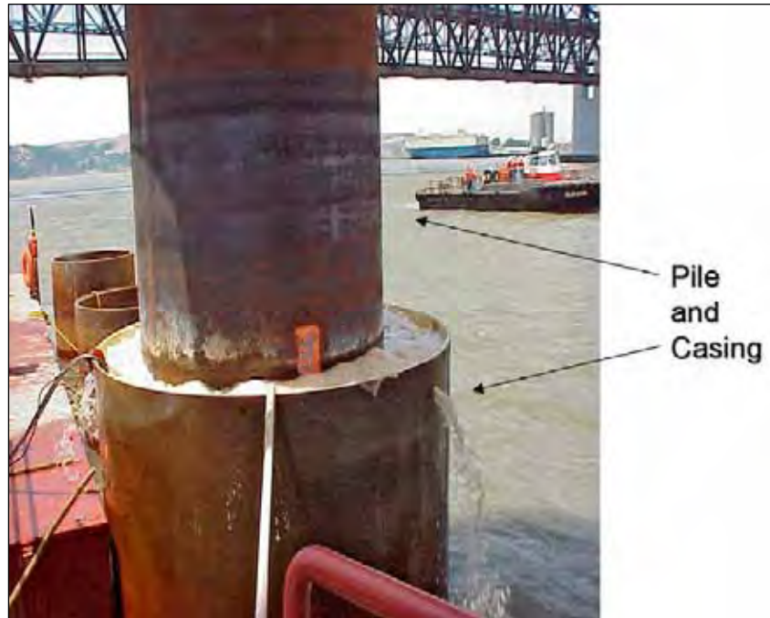
Figure 2-30. Confined Air Bubble Curtain System Used in an Isolation Pile at the Benicia-Martinez Bridge
