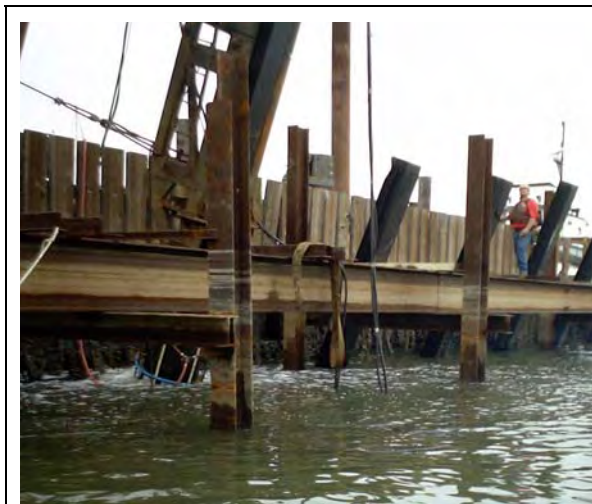
Figure I.4-2a Impact Driving of Battered H-Type Pile with Attenuation System, with Vertical Thin-Walled H-Type Piles in Foreground
