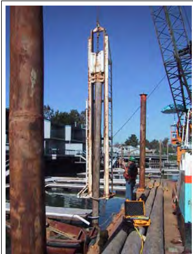
Figure I.7-1 Driving of Timber Piles at Ballena Bay Marina Using a 3,000-Pound Drop Hammer
