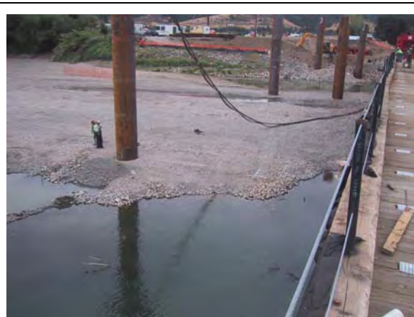
Figure I.3-22a Vibratory Installation of a Bent 4 Pile with Bent 3 and Bent 2 in the Background
