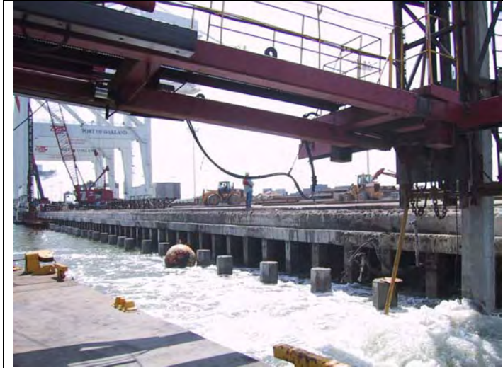
Figure I.5-12 Driving of 24-Inch Octagonal Piles at Berth 32, Port of Oakland with an Air Bubble Curtain System to Attenuate Sounds
