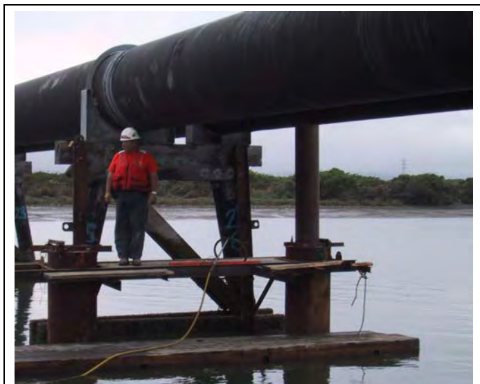
Figure I.3-3 Installation of 13-Inch-Diameter Steel Pipe Piles with Confined Air Bubble Curtain System
