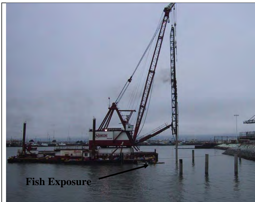
Figure I.5-9 Pile Driving during Fish Exposure Study at Berth 22, Port of Oakland. Picture was taken 100 meters west of pile driving activity, while fish were being exposed at 10 meters from the pile.
