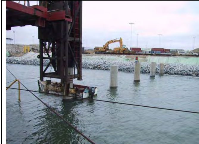
Figure I.5-6 Driving of 24-Inch Octagonal Indicator Piles at Port of Oakland Berth 22. Pile being driven is in Row A, while Row E is at the shoreline.
