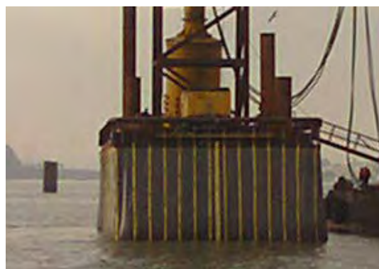
Figure I.9-4b Proprietary Fabric Air Bubble Curtain (Proprietary) Used during Driving of PIDP Pile 3
