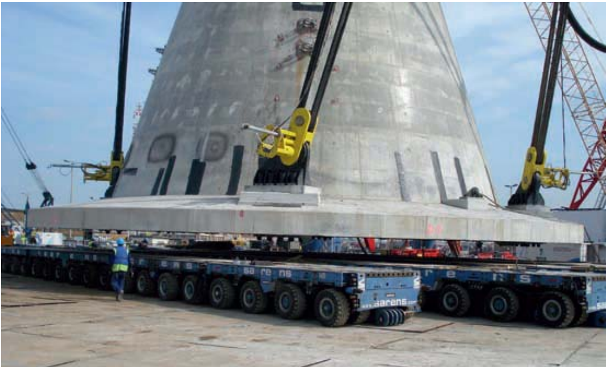
Figure 4-7 Gravity base foundation being prepared for lift-off from the quay (Source: Peire et al. , 2009)
