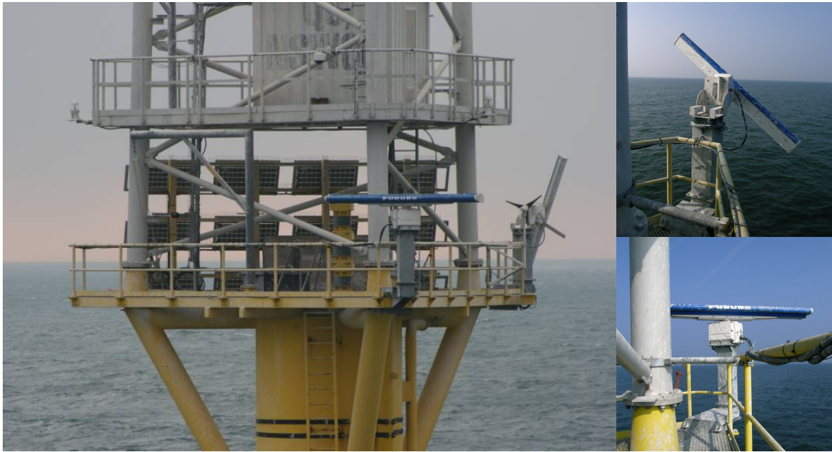
Figure 9. Merlin Radar at the OWEZ metmast, overview and details of vertical and horizontal radar respectively (photos M.J.M. Poot and K.L. Krijgsveld).
