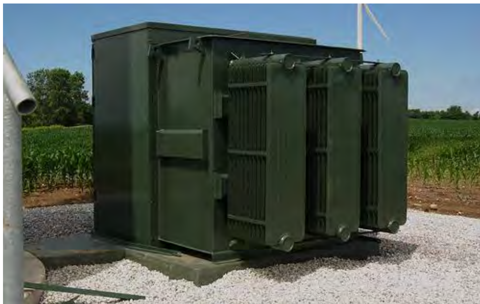
Figure 2-6 Typical Pad-Mounted Transformer
