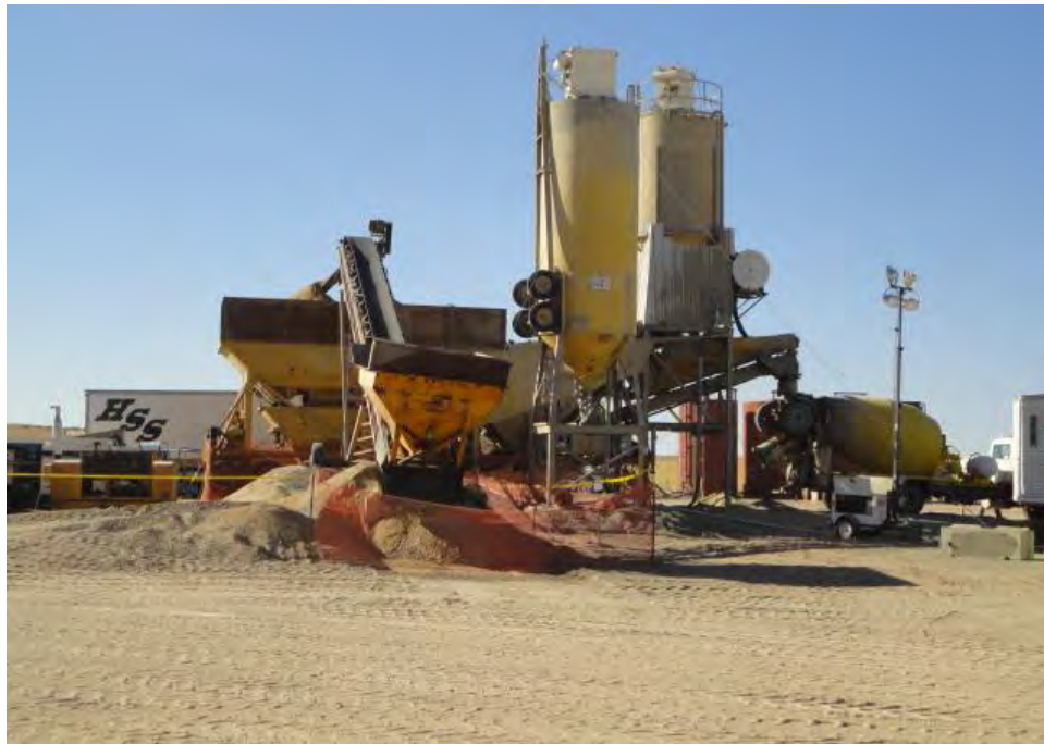
Figure 2-2 Typical Temporary Concrete Batch Plant
