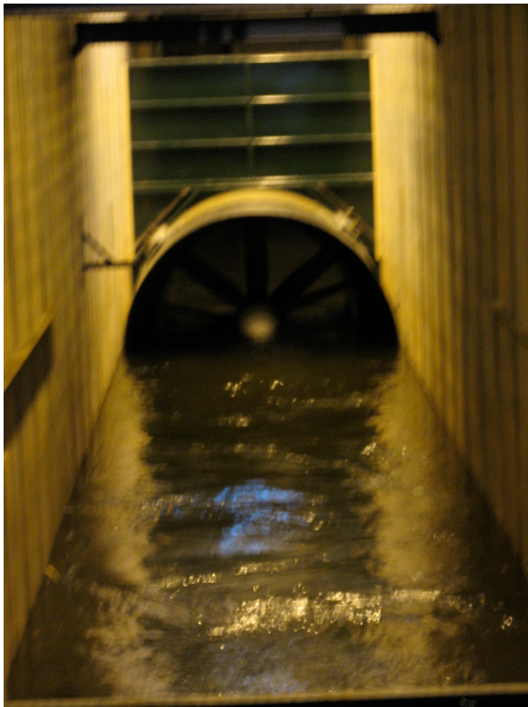
Installed in Test Flume
