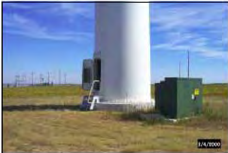
Pad Transformer at Base of Turbine
