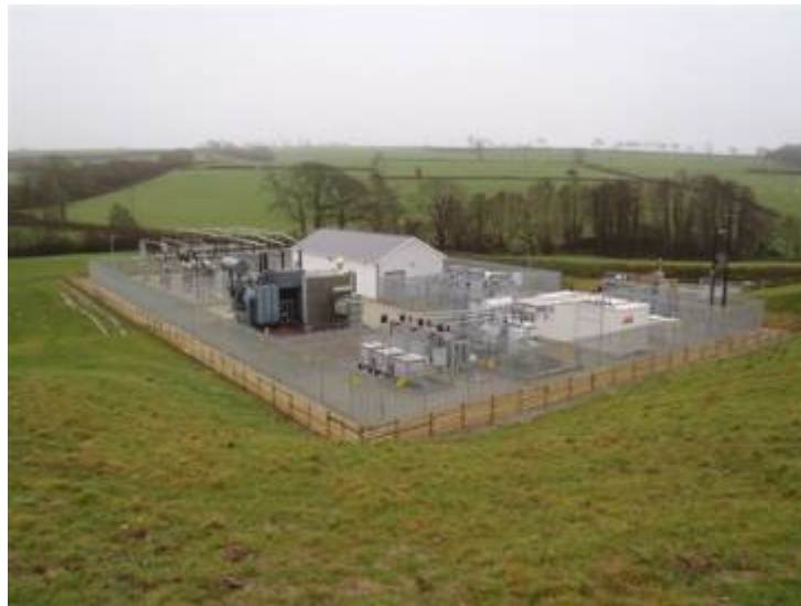
Figure 5.15: Typical 33/132kV Sub-station/Control Building
