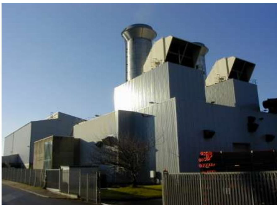
Figure 4.14 – Guernsey's main power station at St Sampson's (photo – GEL)
