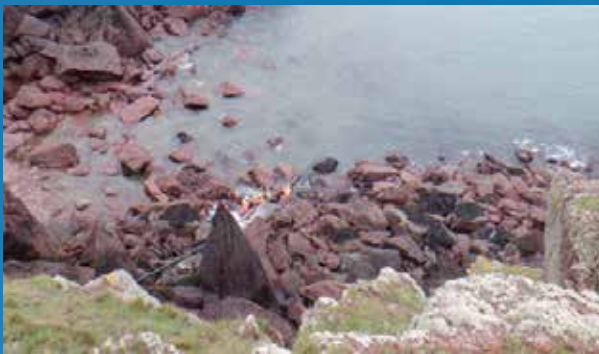
Conduit installation at East Pickard Bay where mWave demonstrator cable lands ashore
