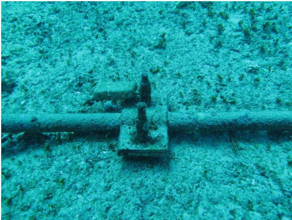
Figure 15. Power cable at approximately right angle in the same location in May 2011. Note, greater abundance of Halimeda sp. in 2011 and coral growing on anchor bolt
