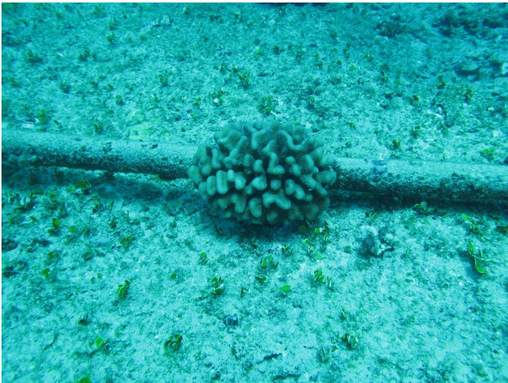
Figure 17. Power cable in 2011 at approximately 50 ft
