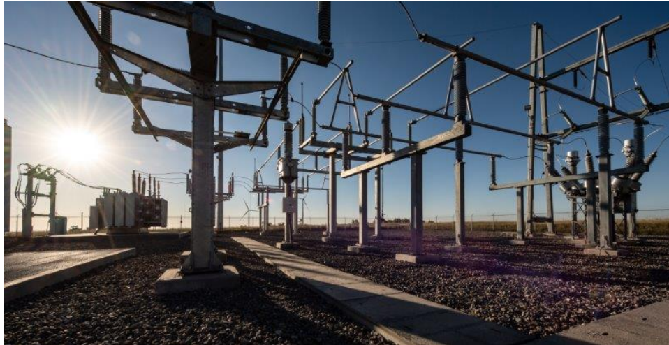
The Flatirons Campus substation at NREL is part of the Power Generation Upgrade Project, which is changing the source of utility power at the Flatirons Campus from the distribution network that feeds businesses and houses to the transmission network that ties all the power plants and substations together. Photo by Dennis Schroeder, NREL
