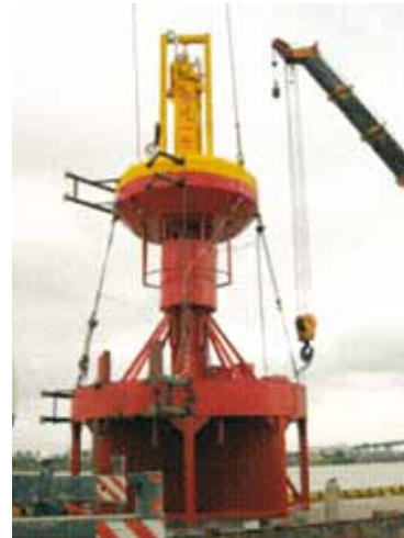
Installation of the 10kW prototype testing (GIEC of Chinese Academy of Sciences)
