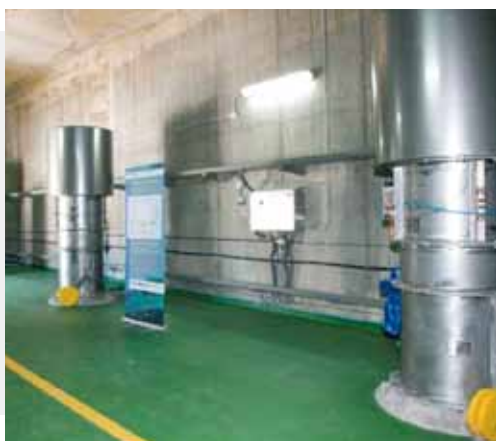
Turbines of the Mutriku OWC plant
