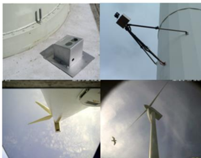
Figure 12 WT-Bird system installed on a wind turbine in Den Helder (images taken from Verhoef et al., 2004)
