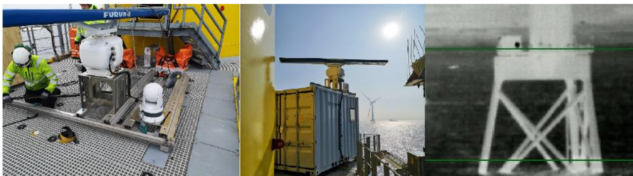
Figure 11 MUSE system installed at Aberdeen European Offshore Wind Deployment Centre (images taken from DHI MUSE website)
