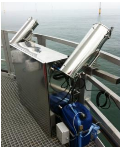
Figure 17 ACAMS installed offshore (image taken from Dirksen, 2017)
