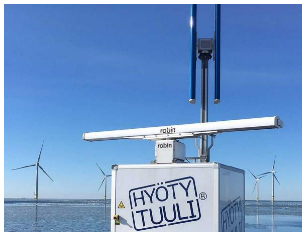
Figure 4 Robin Radar installed at Tahkoluoto wind farm, Finland (image taken from Robin Radar, 2021)
