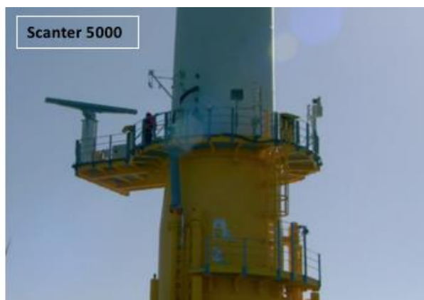
Figure 2 SCANTER-5000 Radar installed on Turbine G01 at Thanet offshore wind farm (image taken from Skov et al., 2018)
