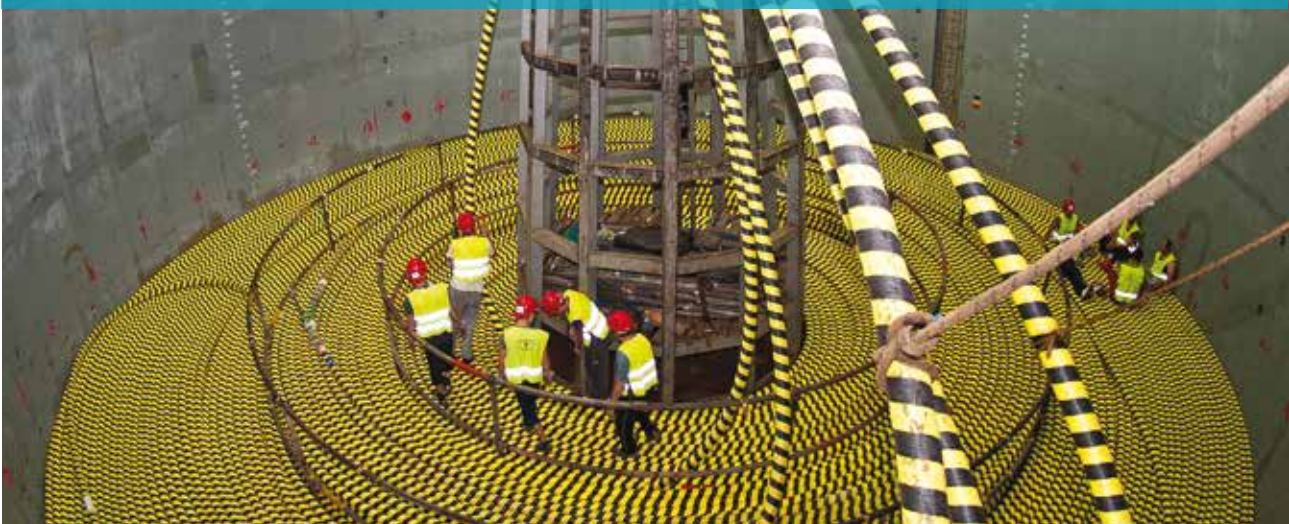
Image of cable drum housing EMEC cable by Mike Brookes-Roper
