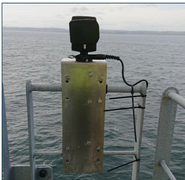
Figure 3-6 The R-Vision SeeHP camera in position at AWF6, EOWDC
