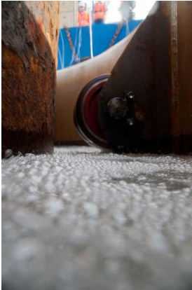
Figure 13: View of the gap between the pile/NMS during operation of the bubble curtain (photo: Patrice Kunte)
