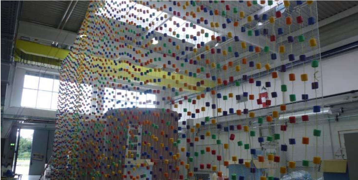
Figure 29: Constructing the middle net with HSD foam elements (source: TU Braunschweig/Dr. Elmer)
