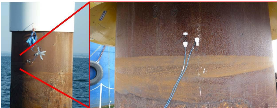
Fig. 1: Measuring positions of the acceleration sensor (right) and expansion sensor (left) at the Brodten Pile
