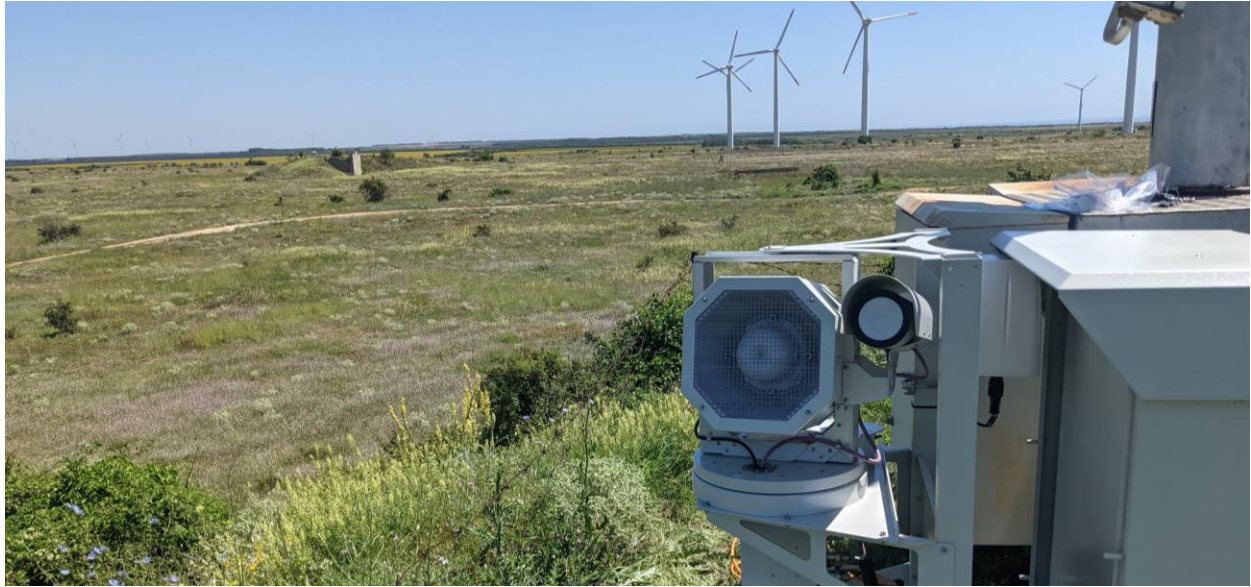
Figure 3. Volacom's BCAS, installed in the Kaliakra region, NE Bulgaria.
