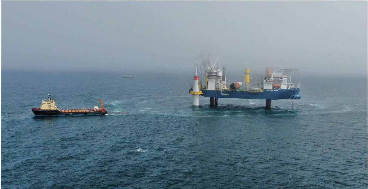
Figure 2.2 The double Big Bubble Curtain (dBBC), deployed and operated from the M/V Commander, during the installation of monopile A02.
